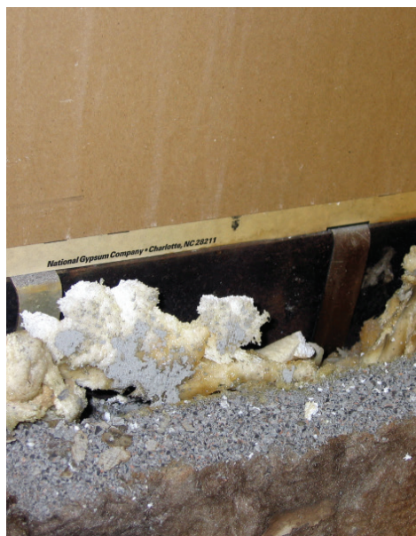
The Gypsum beneath the ProGUARD® is completely free of smoke or fire damage.
