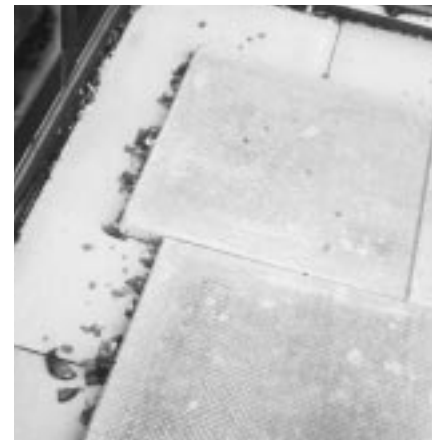
As you can see for yourself, LIGHTGUARD protects the waterproof membrane from punctures caused by dropped tools, vandalism or even this broken pop bottle found on the N.E. Clinton School.
