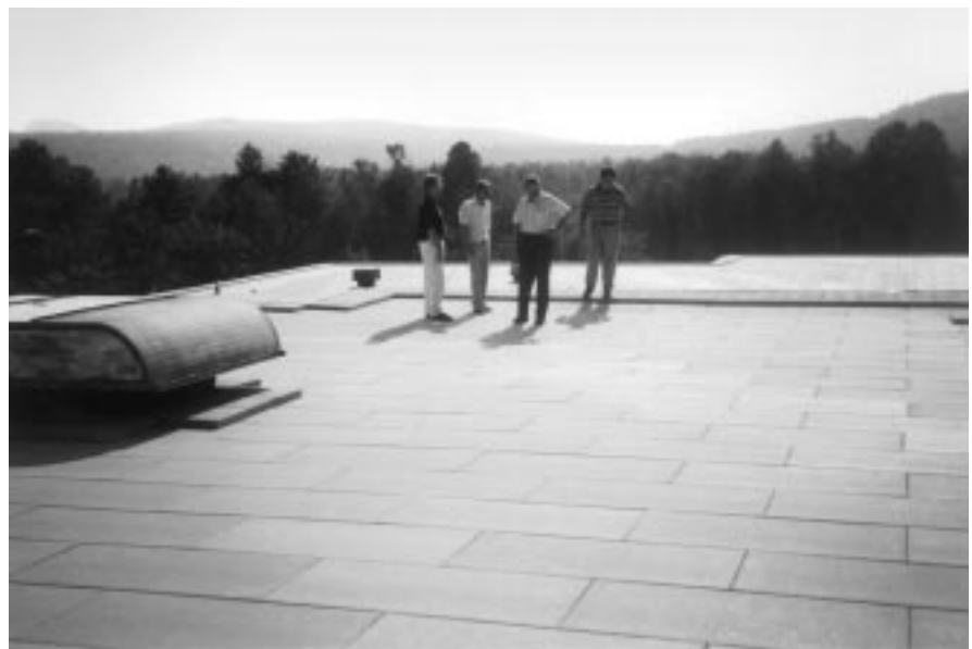
L to R: T. Clear approved contractor Mike Monahan, Pres. Monahan & Loughlin, Inc.; T. Clear agent Ken Ross, Pres. Styro Moisture Protection; Randy Windell, V.P. /General Manager, T. Clear Corp.; Brian Monahan, Supervisor, Monahan & Loughlin, Inc. standing on a LIGHTGUARD Protected Membrane Roof System atop the Ausable Valley Middle High School .
