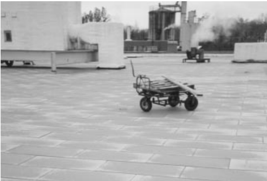
A view of the latest LIGHTGUARD section with a typical maintenance cart. Showing are just a few of the many penetrations at The New Cherokee Corp.
